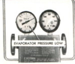
FIGURE 7—TXV STUCK CLOSED
