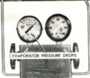
FIGURE 5—POA VALVE STUCK OPEN
